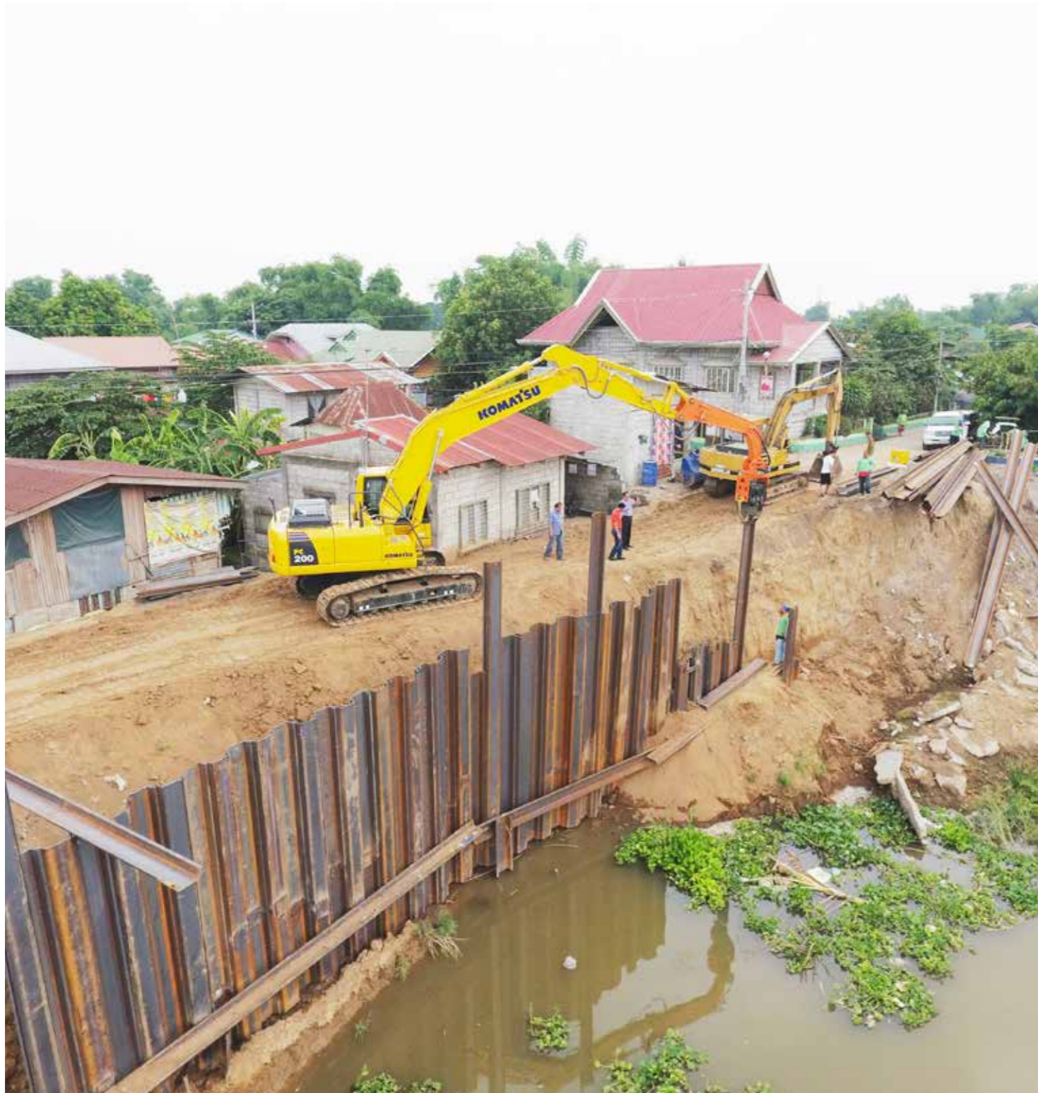
Dike Repair and protection to river bank. Supplied Hot Rolled Sheet Piles
